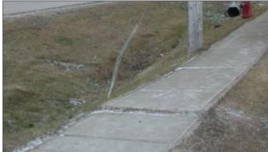
Shifted pavers on this sidewalk create a potential tripping hazard.
